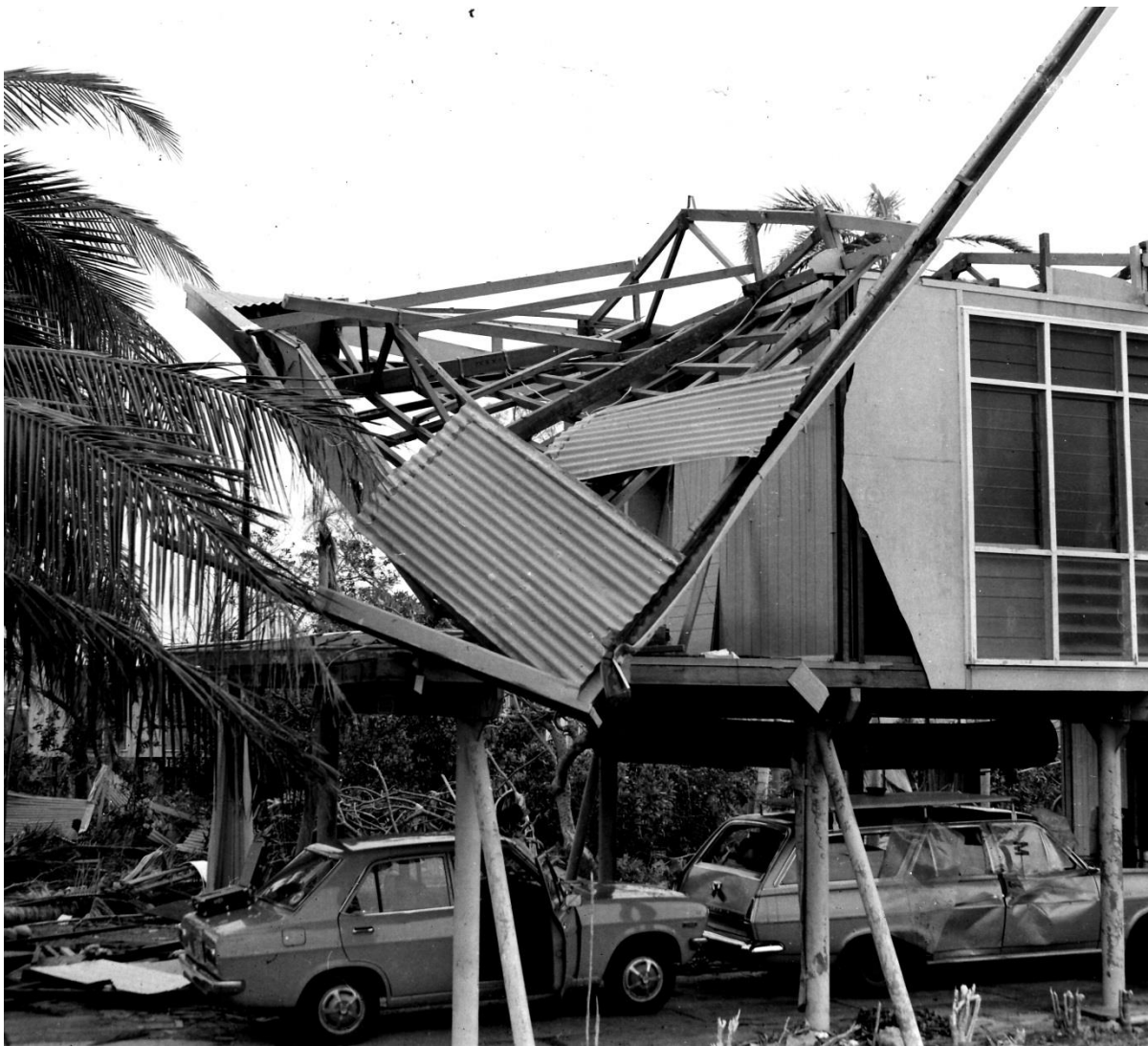
A closer view of the damaged part of 16 Porter Street. Prior to Cyclone Tracy, the vehicles were hidden by a row of Arailia trees (arailia spinosa). In this picture the 'stumps of the trees can be seen. The trees were sheared off by flying corrugated iron.
