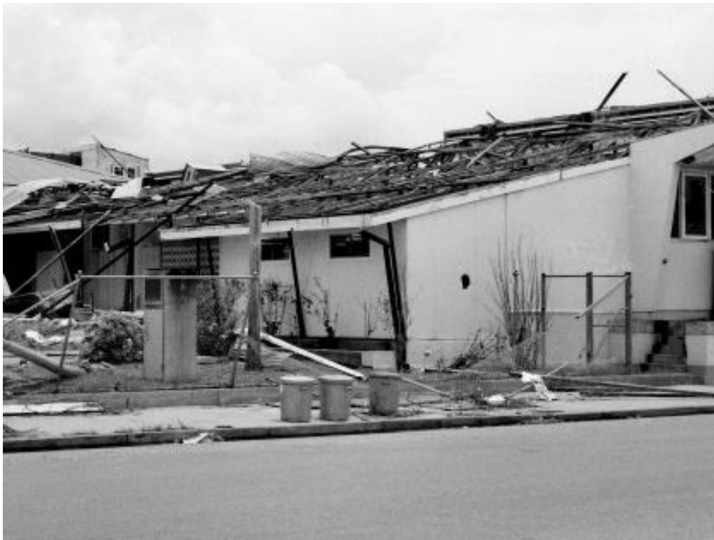
The roof of the Assembly's garden store and printery after the cyclone.
