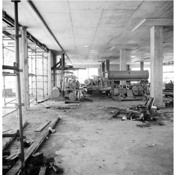
Backup generator waiting to be installed.
